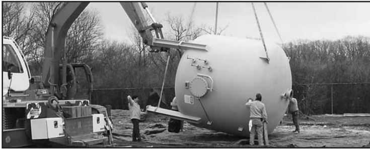
The resin treatment plant being developed at the Bethpage Water District's Plainview Road well site is expected to be operational before the summer season heats up.
